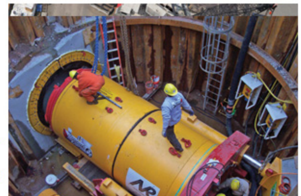
This project is the longest and largest microtunnel project in New Jersey in recent years.
